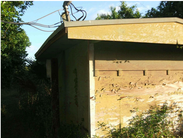
West electric pump house 4
