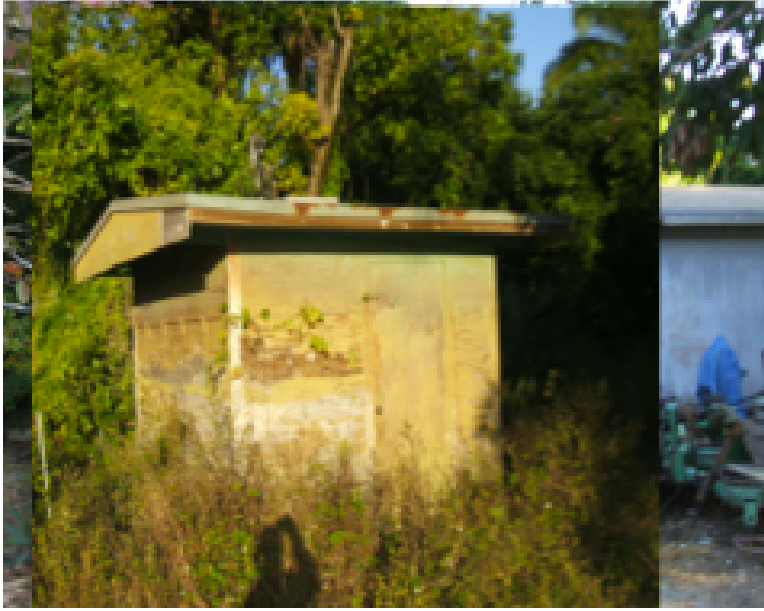
West Electric pump house
