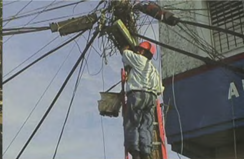
Pirating electricity is a common practice in the developing world, and the pirates make a good living. Unfortunately for the power company workers, like this one in Santo Domingo, they have to sort through the highly charged mess.
