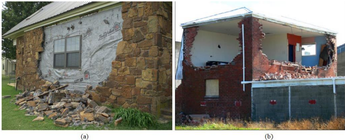
Figure 2.1. Masonry wall damaged by earthquake excitations: (a) the 2016 magnitude 5.8 Pawnee earthquake in Oklahoma (Clayton et al. 2016) and (b) the 2010 magnitude 7.1 Canterbury earthquakes in New Zealand (Dizhur and Ingham 2015); Image reused with the written permission from T. Clayton and D. Dizhur.
