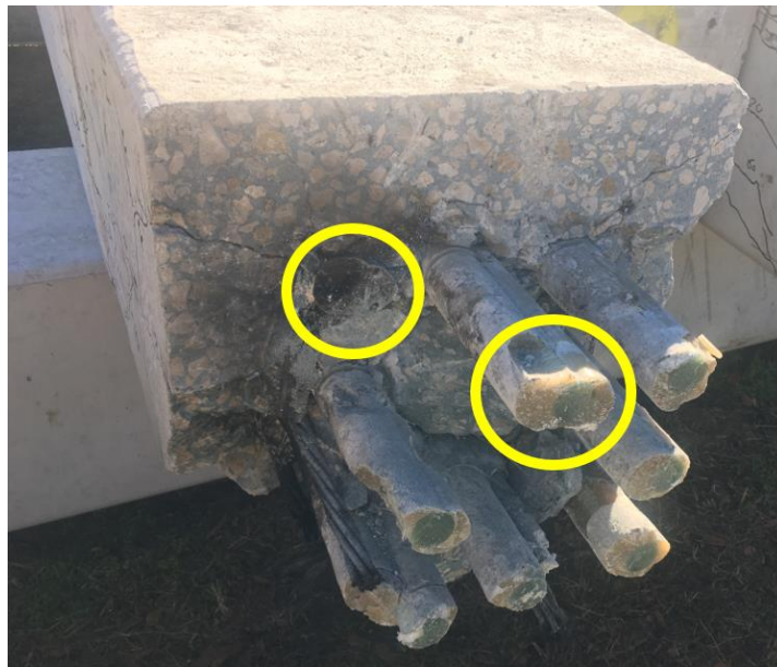
Figure 78: The oversized slanted holes
