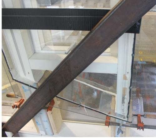
Figure 4.10: Installed plexiglass water collection system
