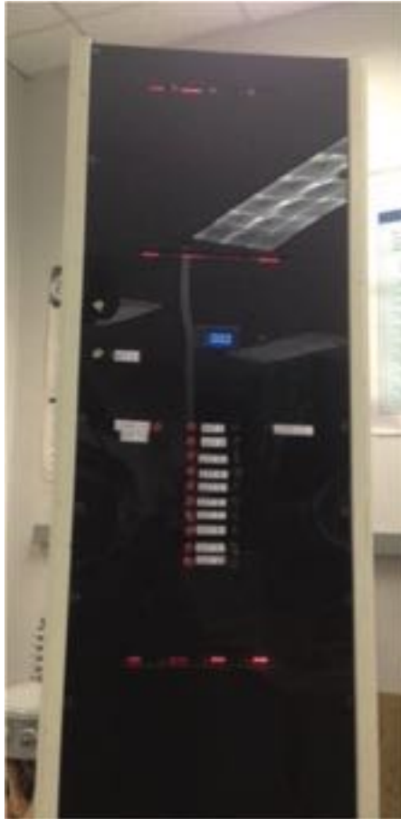
Figure 10.6 Battery Bank Stored Safely in a Closed Cabinet.
