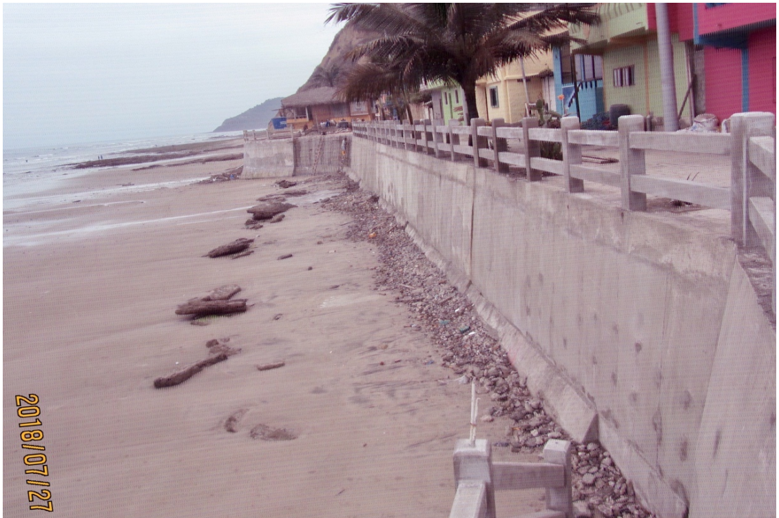
Figure 7. Coastal protection at Comuna La Entrada. Source: Author (2018)
