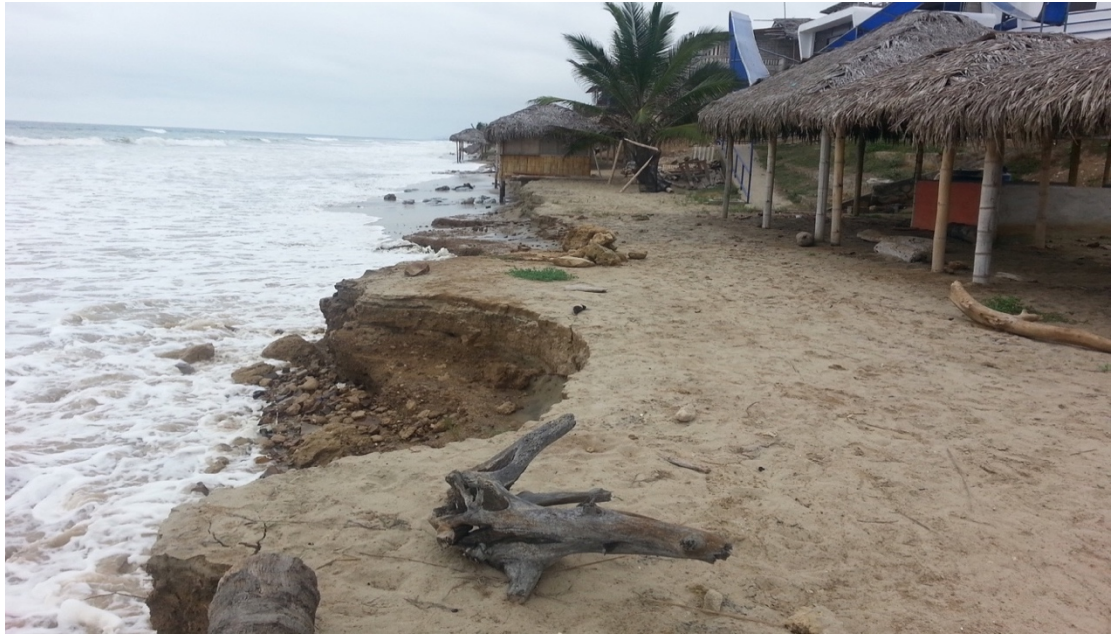
Figure 13. Damages at Libertador Bolívar south beach during November 2015. Source: Enrique Sanchez
