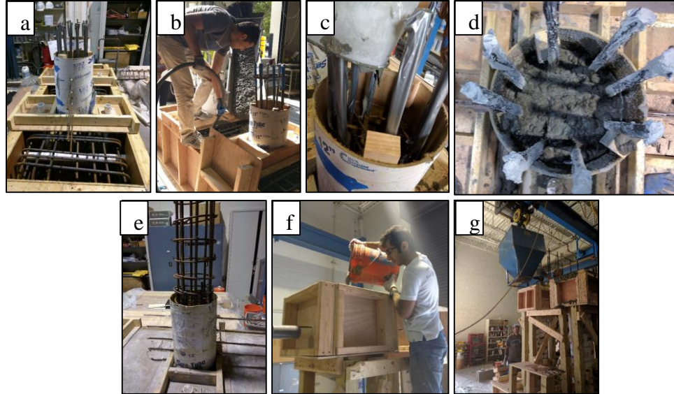
Figure 5-3 Specimen construction procedures a) Formwork of the support, b) Casting support, c) Casting first layer of UHPC, d) Casting plastic hinge, e) Reinforcement of the column, f) Casting splice region with UHPC and g) Casting column with N.C.
