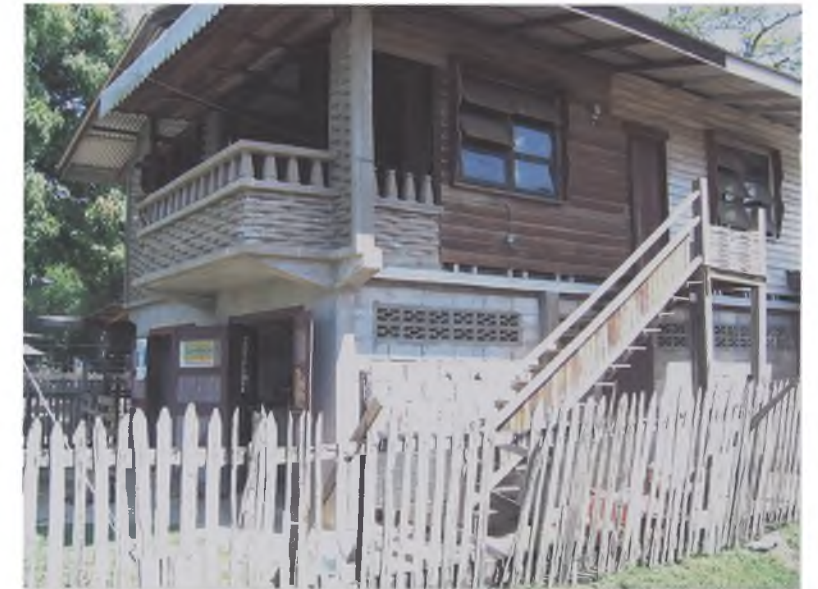
Figure 12: Concrete Addition to Existing Wooden House. The addition is of concrete block construction and is directly attached to the original wooden house.
