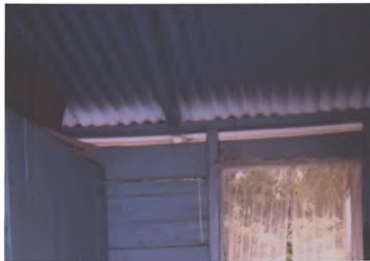
Figure 17a: Interior View of Opening between Roof and Wall. This narrow gap facilitates cooling of interior spaces as well as the roof.
