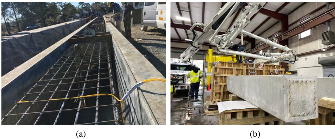
Figure 5.33: Construction of the 30-inch specimens (a) pile casting at CDS, (b) pile cap casting at FDOT SRC
