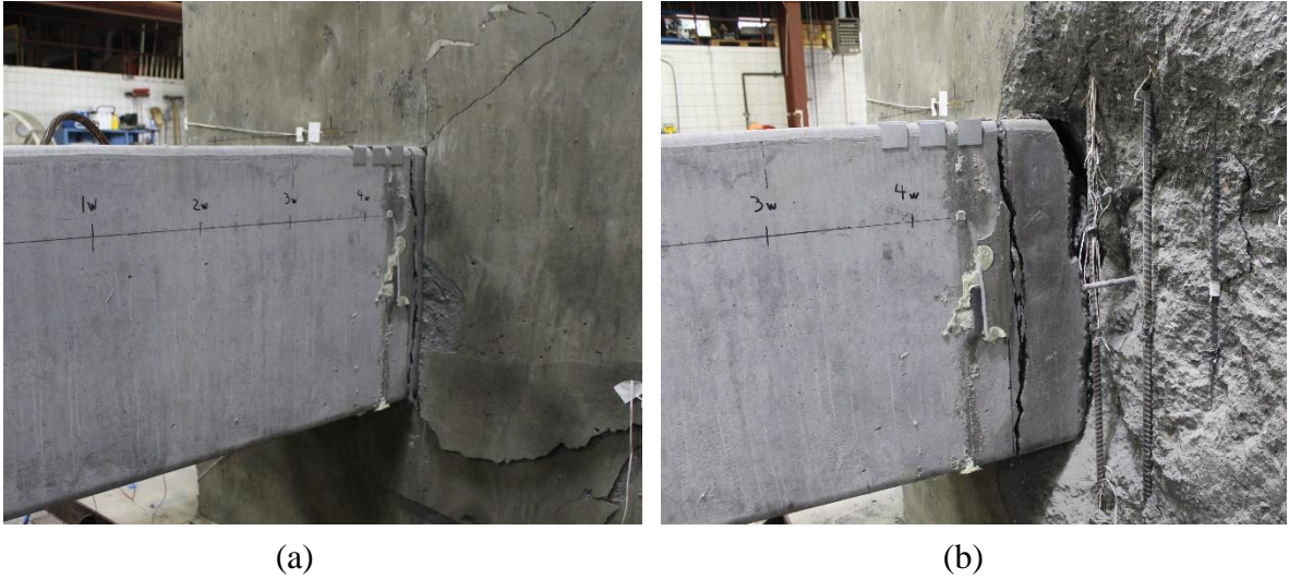
Figure 5.52: SP-09 strand development failure (a) SP-09 failure, (b) after removing spalled concrete in the cap
