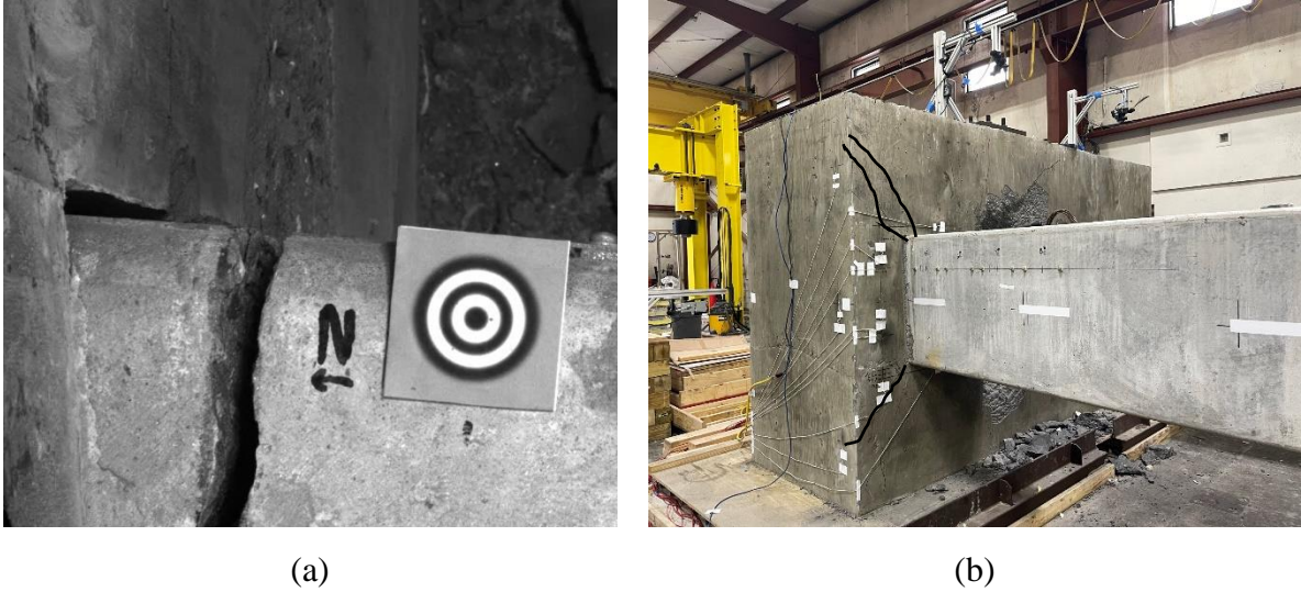
Figure 5.53: SP-09 failure (a) pile slipping out of pile cap (b) damage in pile cap
