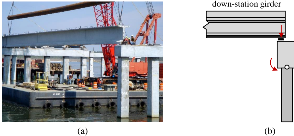
Figure 3.1: (a) Construction of a bridge with tall pile bents (courtesy of Corven Engineering) and (b) schematic of unstable bent with assumed pinned connection
