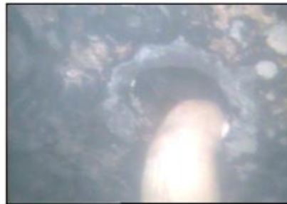
Figure 4.1. Underwater image of a hole on a steel pile due to corrosion. Photo courtesy of FDOT.
