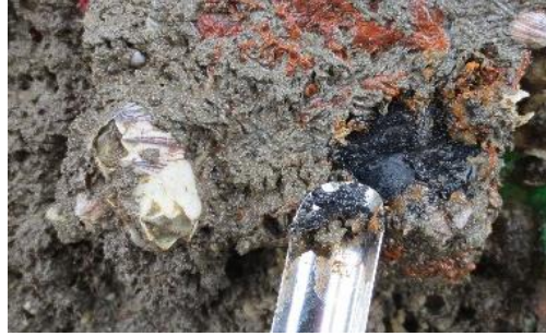
Figure. 5.16. Example of Under Fouling Surface Condition.
