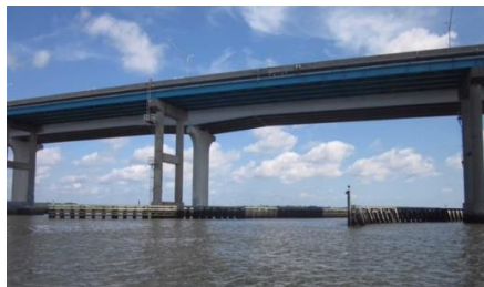
Figure 1.1. Picture of a Florida bridge over Matanzas R. with corrosion of steel piles.
