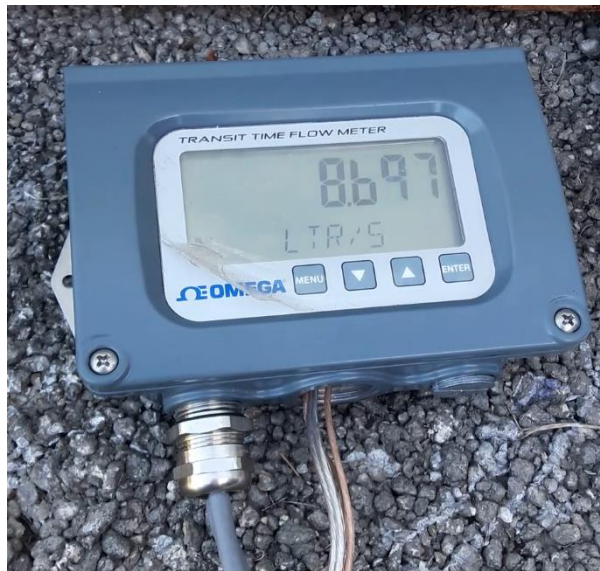
Figure A-4: Omega Flowmeter
