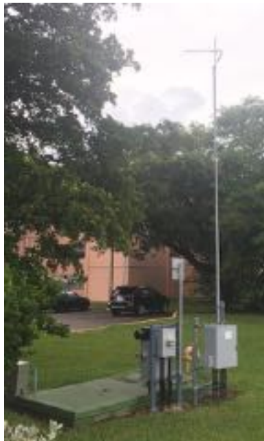
Figure 6 Photo of the antenna in a pump station in Miami, FL that could benefit from a STAR radio.
