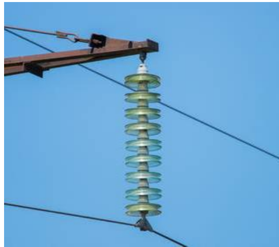
Fig. 1.2: Typical view of an electrical insulator
