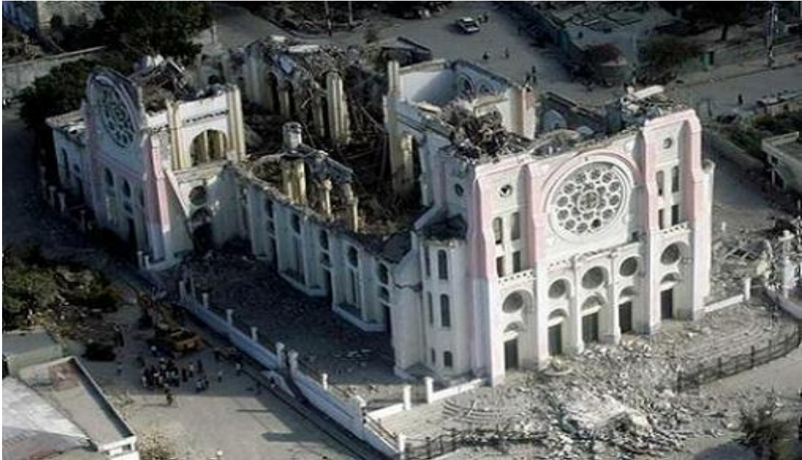
Figure 6.6: Cathedral of Port-au-Prince, Haiti, damaged by the earthquake.
