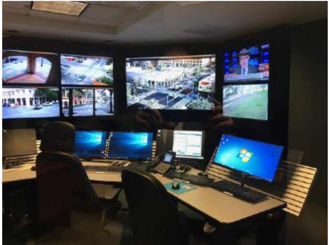
Plate 58. Control office, smart video information. Photograph: Ramon Trias.
