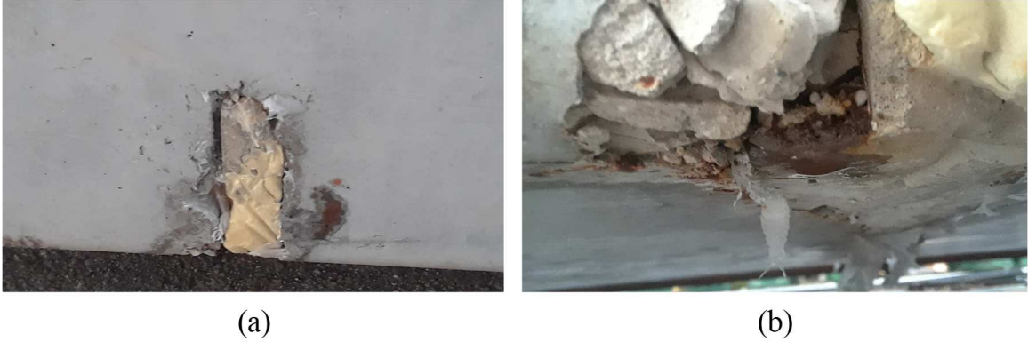
Figure 5-21: Visual corrosion product after accelerated corrosion of Al on FIU-1 on (a) side of beam and (b) bottom of beam
