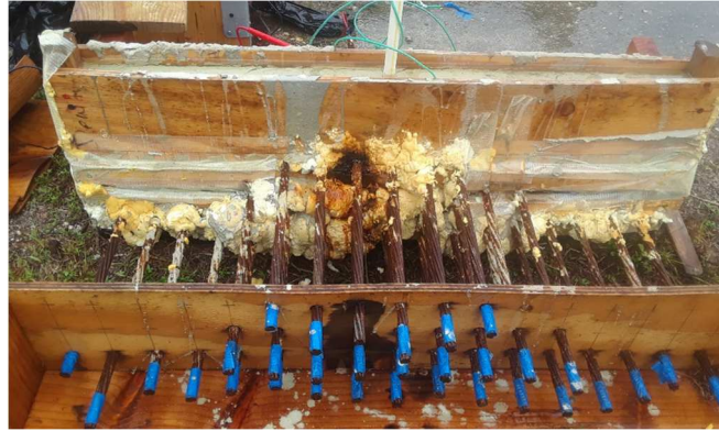
Figure 5-5: Corrosion damage of mockup after 4 days of applying voltage to one of top strands
