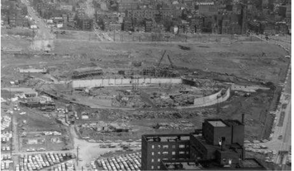
Figure 5.26: Downtown view of Civic Arena construction looking toward the Middle Hill District. Allegheny Conference on Community Development Photographs, MSP285.B001.F17.I03.
