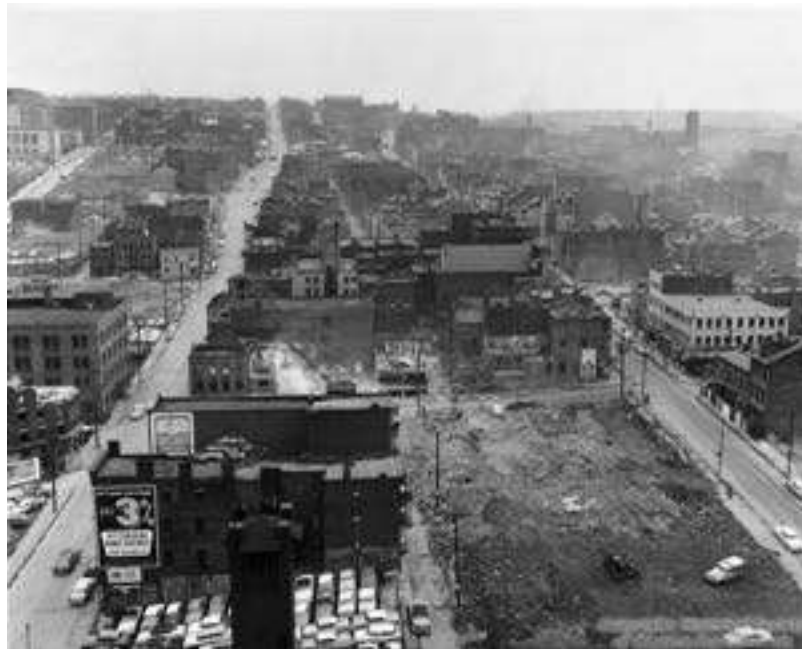
Figure 5.17: Beginning of demolition of the Lower Hill District. Allegheny Conference on Community Development Photographs, MSP285.B001.F17.I02.
