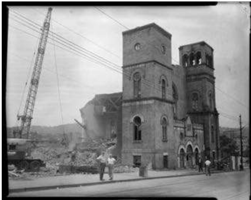
Figure 5.21: Demolition of Bethel AME Church. July 24, 1957. Courtesy of Carnegie Museum of Art, Charles "Teenie" Harris Archive. Accession number: 2001.35.4127.
