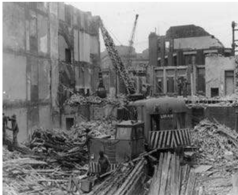
Figure 5.19: Lower Hill District Demolition. Possibly the Musicians’ Clubhouse. Allegheny Conference on Community Development Photographs, MSP285.B033.F07.I02.
