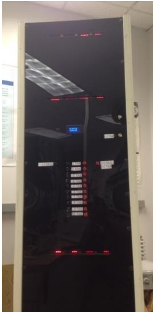
Figure 2.6 Battery Bank Stored Safely in a Closed Cabinet.
