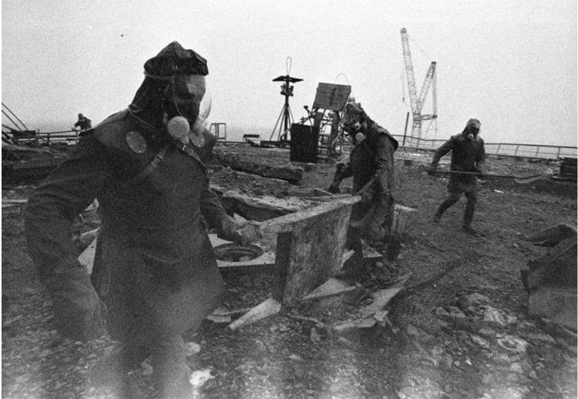
Figure 1.2: Workers known as “biorobots” working on the roof of reactor 3. They would run, remove a few shovels, and then leave. Workers recall feeling pain in their eyes and a metallic taste in their mouth due to the high radiation. [nat11]
