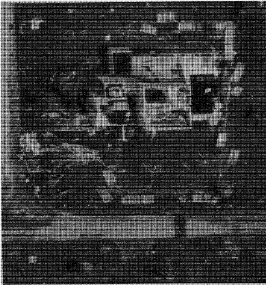
Figure 2.2. Collapse of roof truss.
