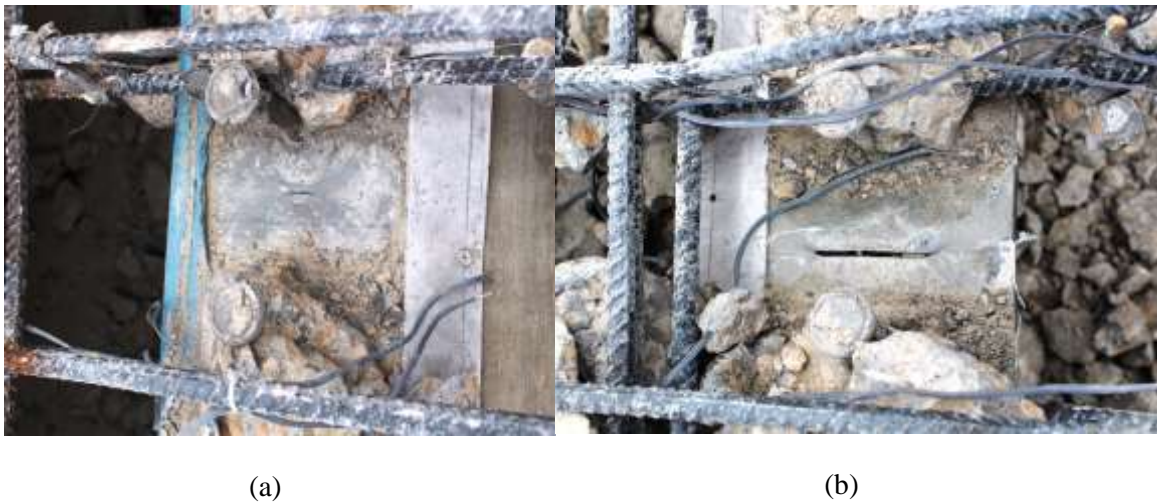
Figure 4-34 Damage in (a) the inner top flange, (b) the outer top flange of the damaged girder.
