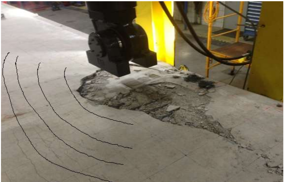
Figure 4-19 Punching in the top of the concrete surface looking to South.
