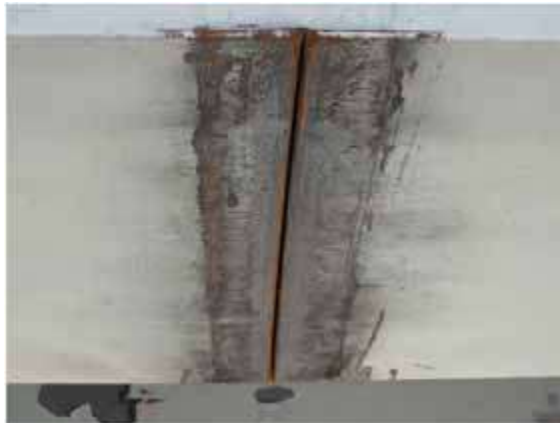
Figure 1-3 Bottom flange cut after the explosion (Source: FHWA Report No FHWA/TX-10/9-5498-1).
