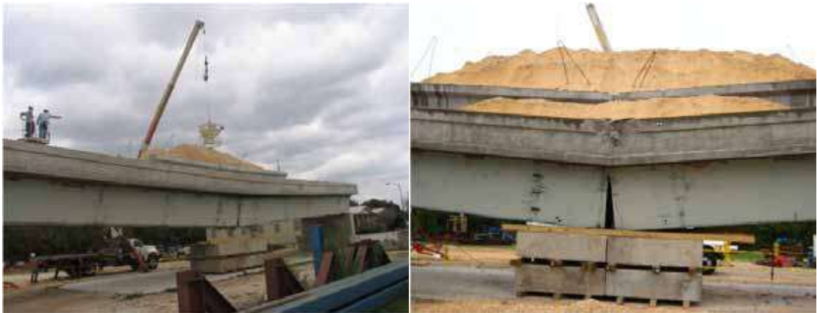
Figure 1-5 FSEL third bridge fracture test (Source: FHWA Report No FHWA/TX-10/9-5498-1).
