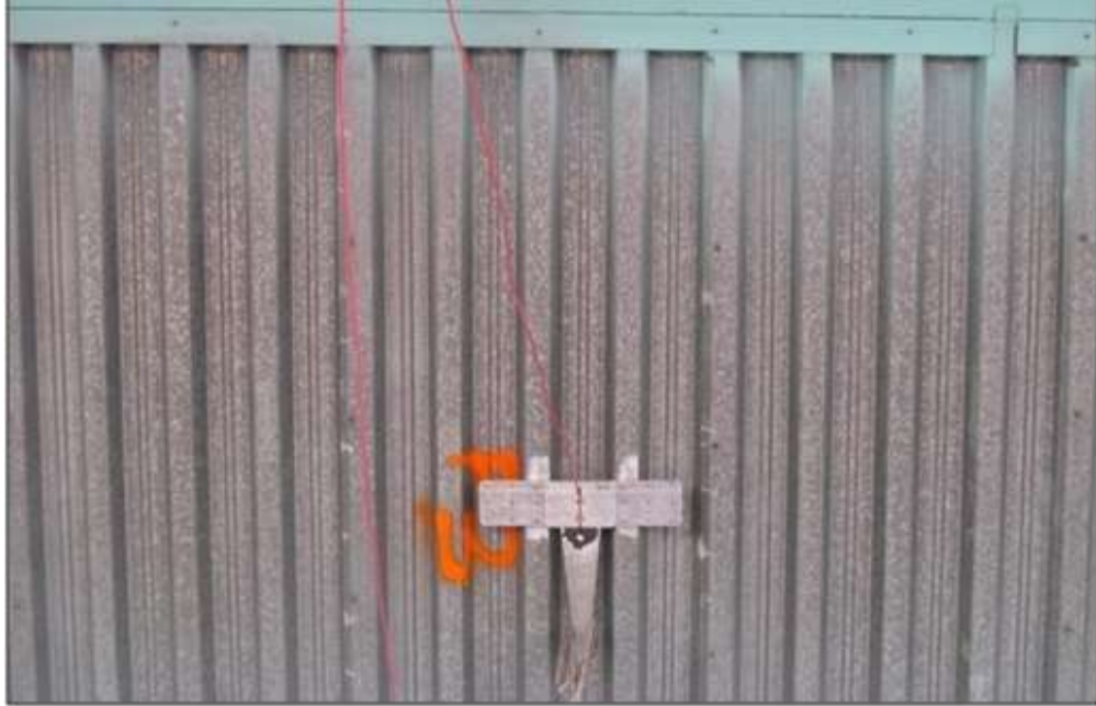
Figure 7-10 Displacement sensor on SIP form below concrete deck.
