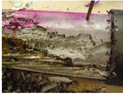
Figure 2.2: Corrosion of Strand Embedded in Deficient Grout. Pink color shows phenolphthalein indicator sprayed on grout surface. Courtesy by FDOT
