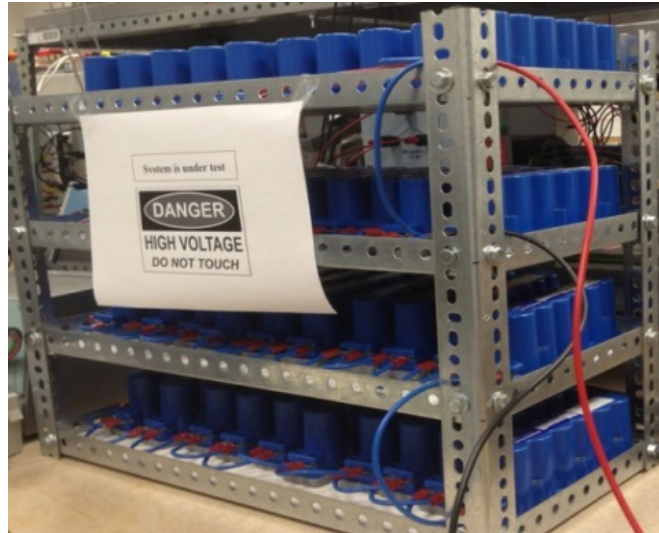
Figure 3.1: Supercapacitor bank setup.
