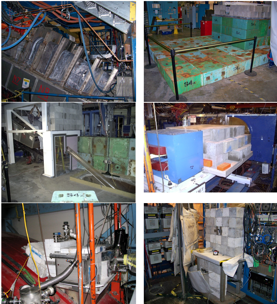
Figure 3.18: Photographs taken after the completion of beamline shielding work. Top left: tagger vacuum box shielding with lead sheet. Top right: Tagger bunker shield. Middle left: Shielded tagger vacuum box and beam dump area. Middle right: The region between the first Italian dipole and the PS dipole. Bottom left: photon collimator shielding area. Bottom right: protective shielding for electronic devices.
