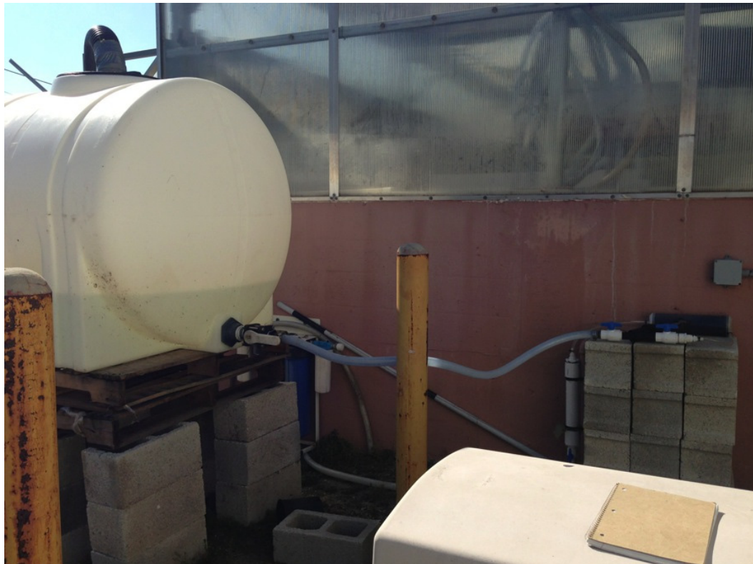
Fig 2. Water filtration system to remove lead (Pb) from the water from hydroponic tanks including holding tank, organics filter and lead (Pb) filter
