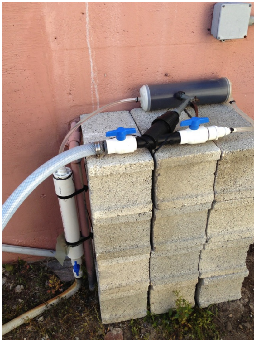
Fig 3. Close up of organic filter and lead (Pb) filter for water from hydroponic reservoir tanks
