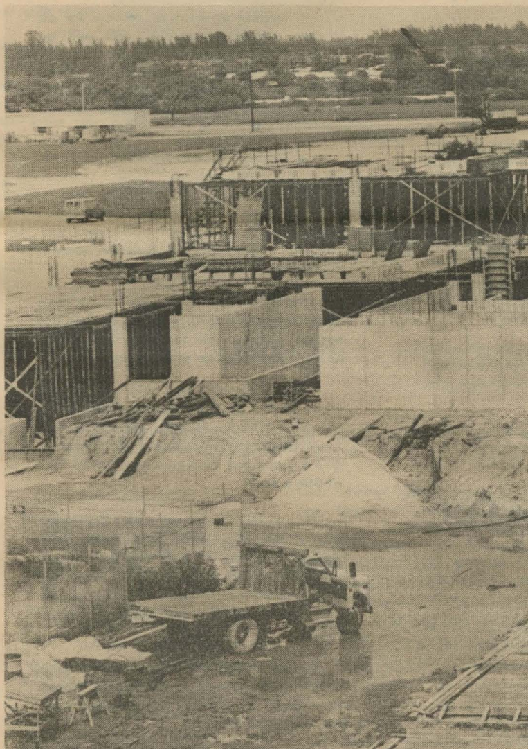
Second Floor Rises — on the new University Services building scheduled for completion in March. The edifice will house the Student Services division, student activities and organizations, cafeteria and rathskeller. (See story page 3)
