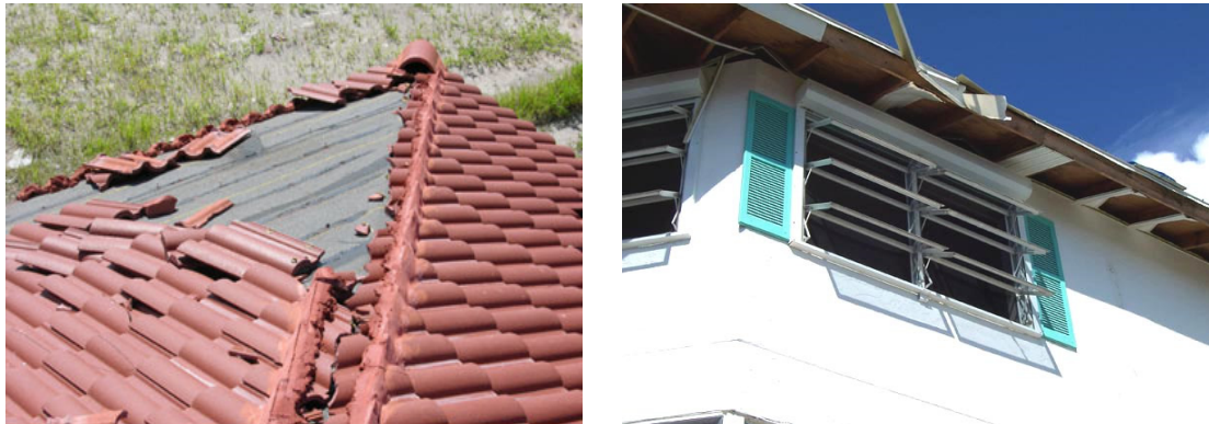
Figure 1.3: Hurricane-induced Damage to Building Envelopes.
