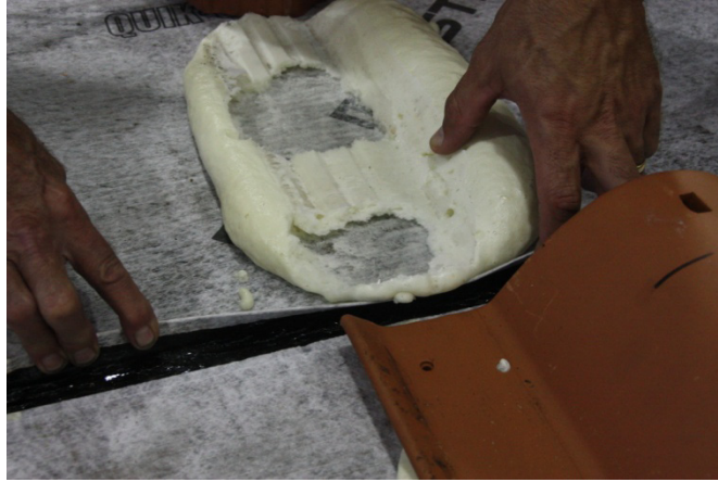
Figure 7.15: Underlayment Detachment from the Deck (Spanish 'S' tile)
