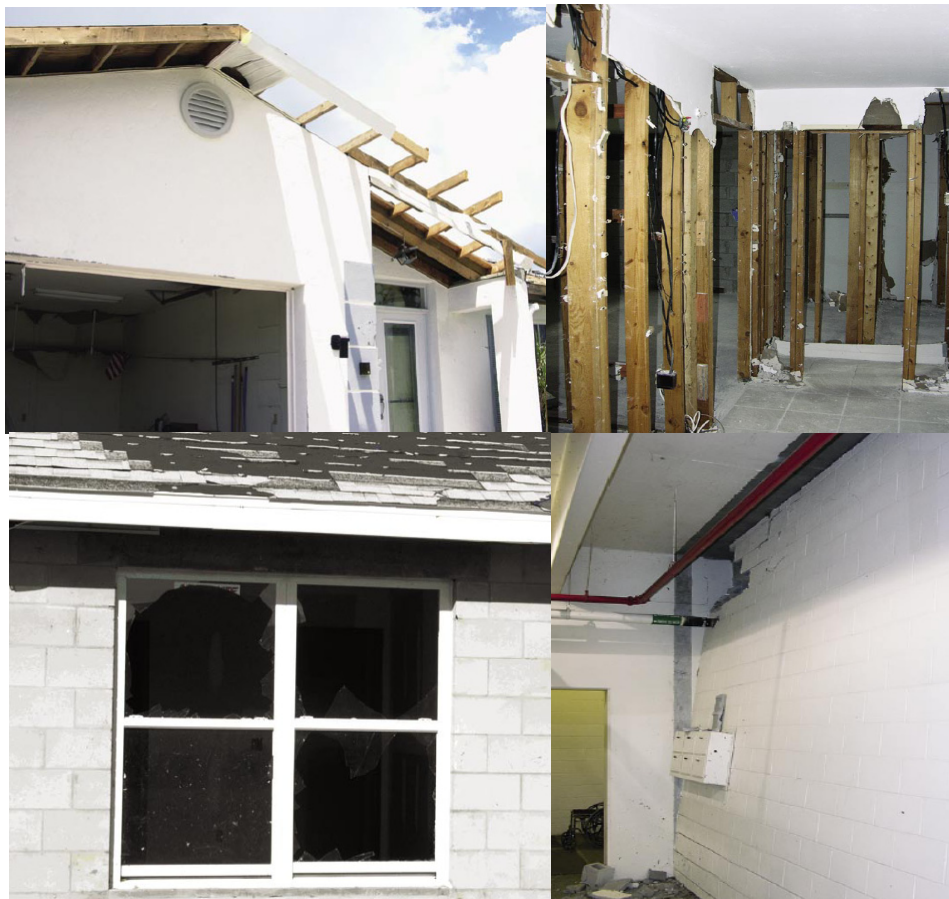
Figure 1.1: Wind induced damage: a) Roof deck failure due to uplift force; b) interior damage due to wind driven rain; c) windows damage by windborne debris; d) internal pressure damage due to failure of external door causing the partition wall to tilt. (Hurricane Charley in Florida, FEMA , 2006)
