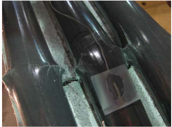
Figure 6.13 Un-cracked Tension Face
