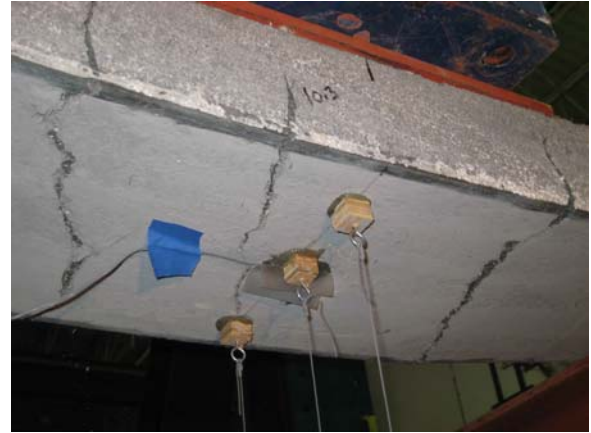
Figure 6.6 Flexural Cracks near Ultimate Load
