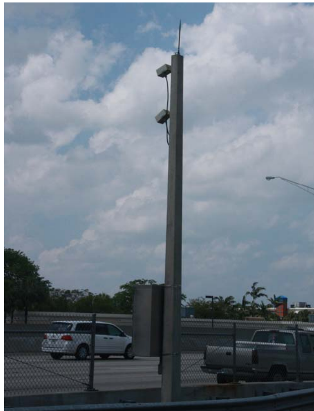
Figure 3-2 Example of Microwave Detectors
