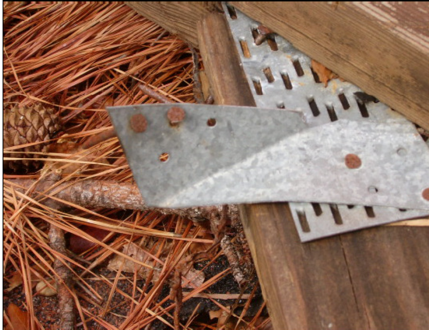
Figure 1-4 Failure of Hurricane clip connecting roof truss and wall with a corroded nails (Van de Lindt, 2005)
