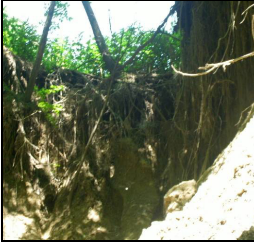
(A) Slumping top of ravine
