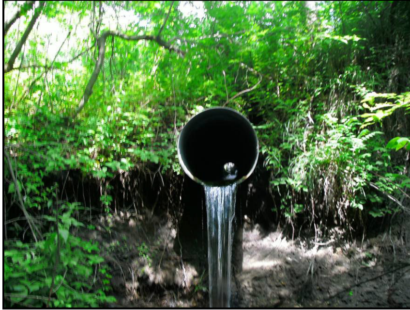
(B) A tile draining water from the collector drain in to a ravine
