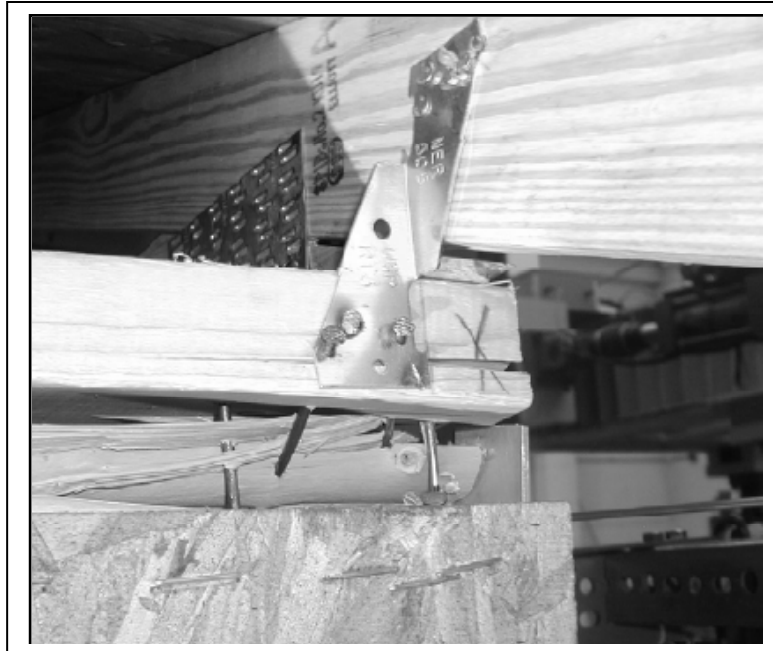
Figure 2.12: Typical Failure Modes of Roof-To-Wall Connections from NIST Tests (NIST, 2003)
