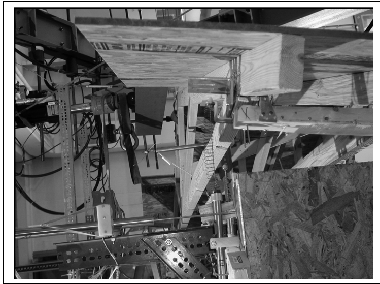
Figure 2.14: Outer Truss Failure Due to Overturning Moment (NIST, 2003)
