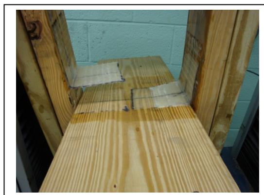
Figure 4.15: Typical Mode of Failure under Lateral Loading (Canbek, 2009)
