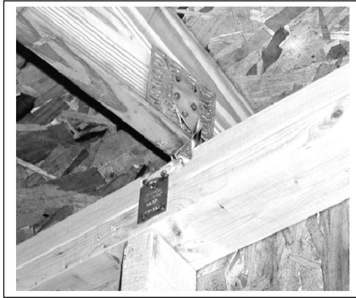
Figure 2.22: Hurricane Clip Tension Failure (NAHB, 2002)
