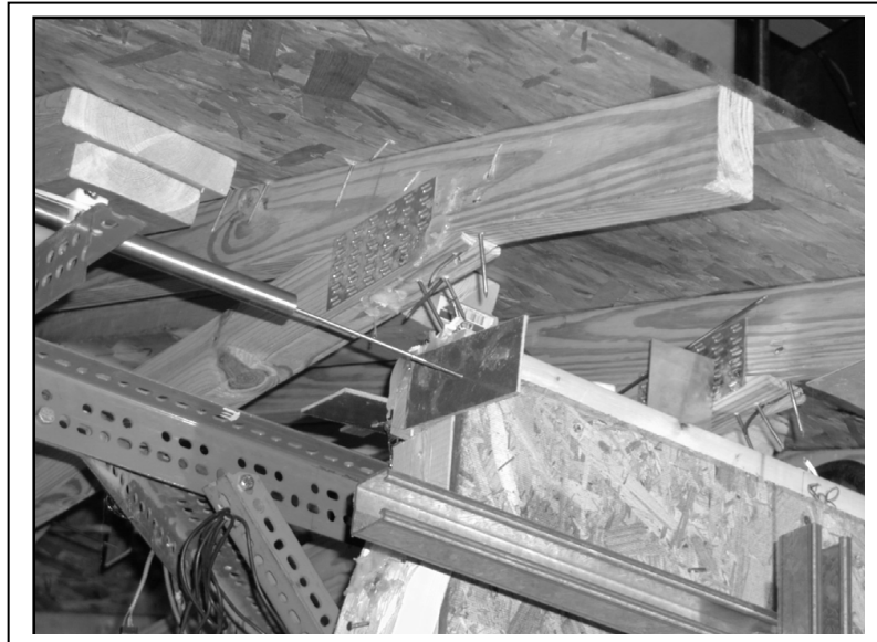
Figure 2.11: Failure of Toe-Nailed Connection with Combined Load (NIST, 2003)
