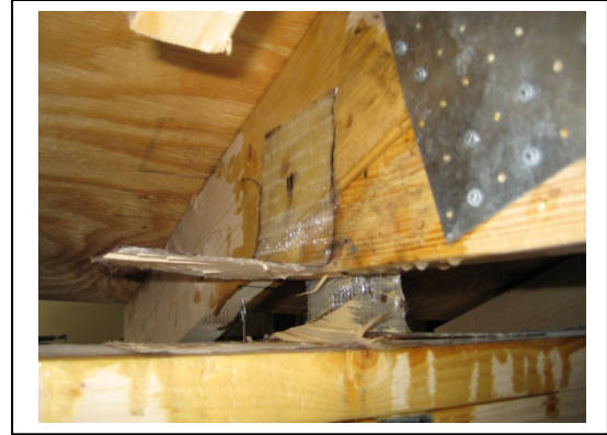
Figure 4.31: Complete Failure of FRP Tie Connections 13 and 14 at 23,659 lbs (Canbek, 2009)
