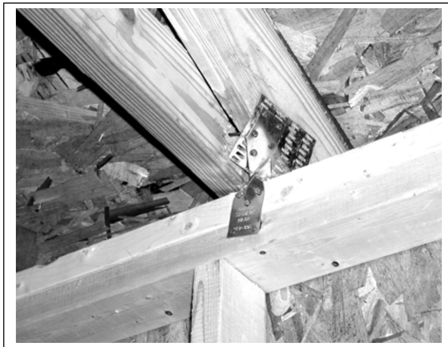
Figure 2.19: Truss Plate Separation (NAHB, 2002)
