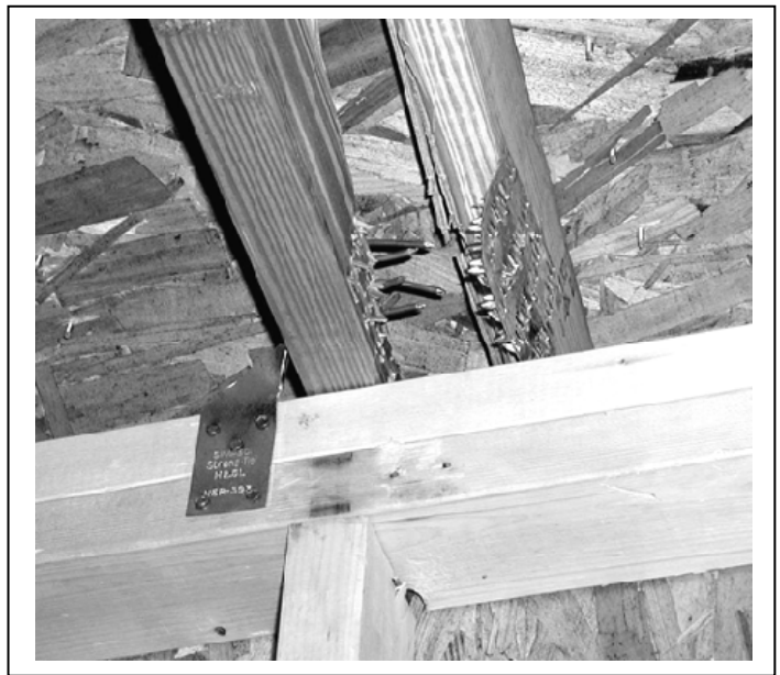
Figure 2.23: Hurricane Clip Tension Failure and Connector Plate Nail Withdrawal (NAHB, 2002)
