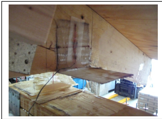
Figure 4.32: Failure of FRP Tie Connections 11 and 12 (Canbek, 2009)
