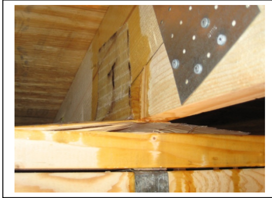
Figure 4.30: Initiation of Failure in FRP Tie Connections 13 and 14 at 20,716 lbs (Canbek, 2009)
