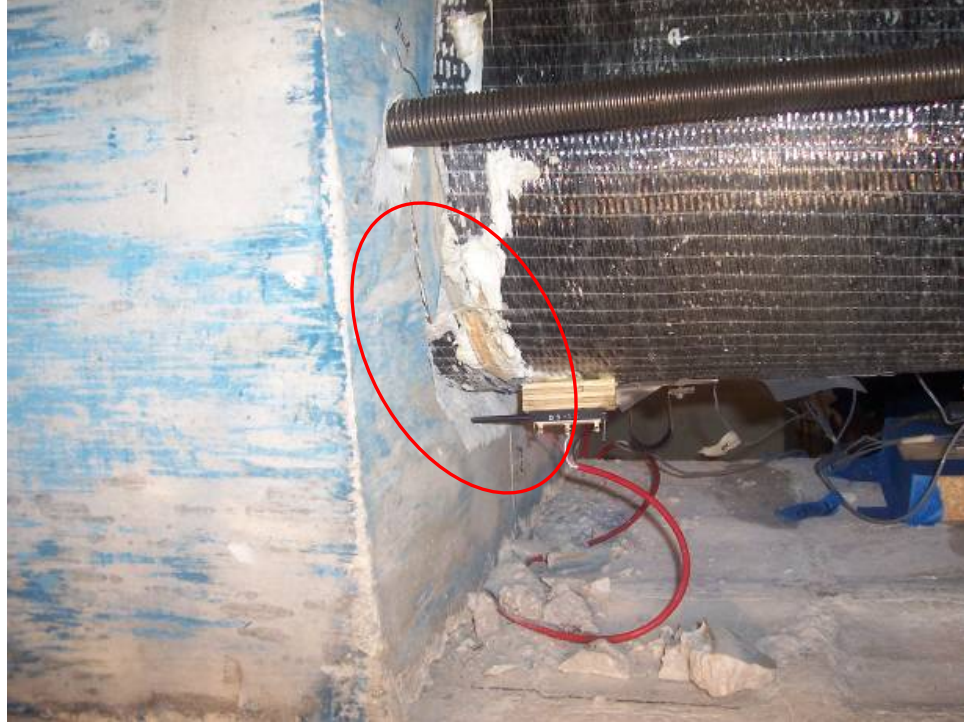
Figure 3.36 Concrete Spalling in Footing of Specimen H
