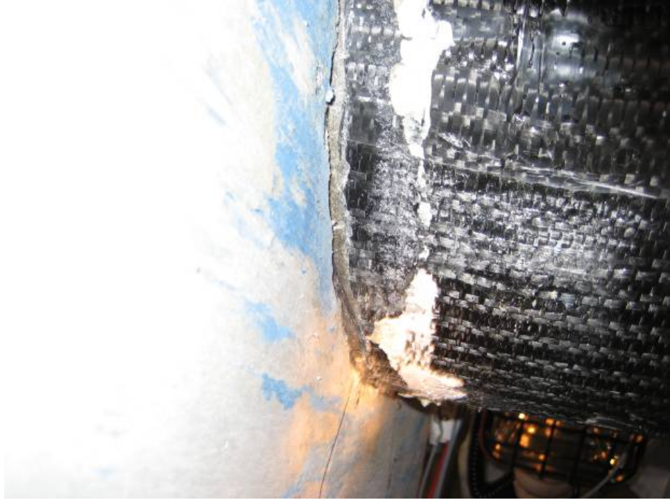
Figure 3.30 Bottom Fiber Crack in Specimen SC
