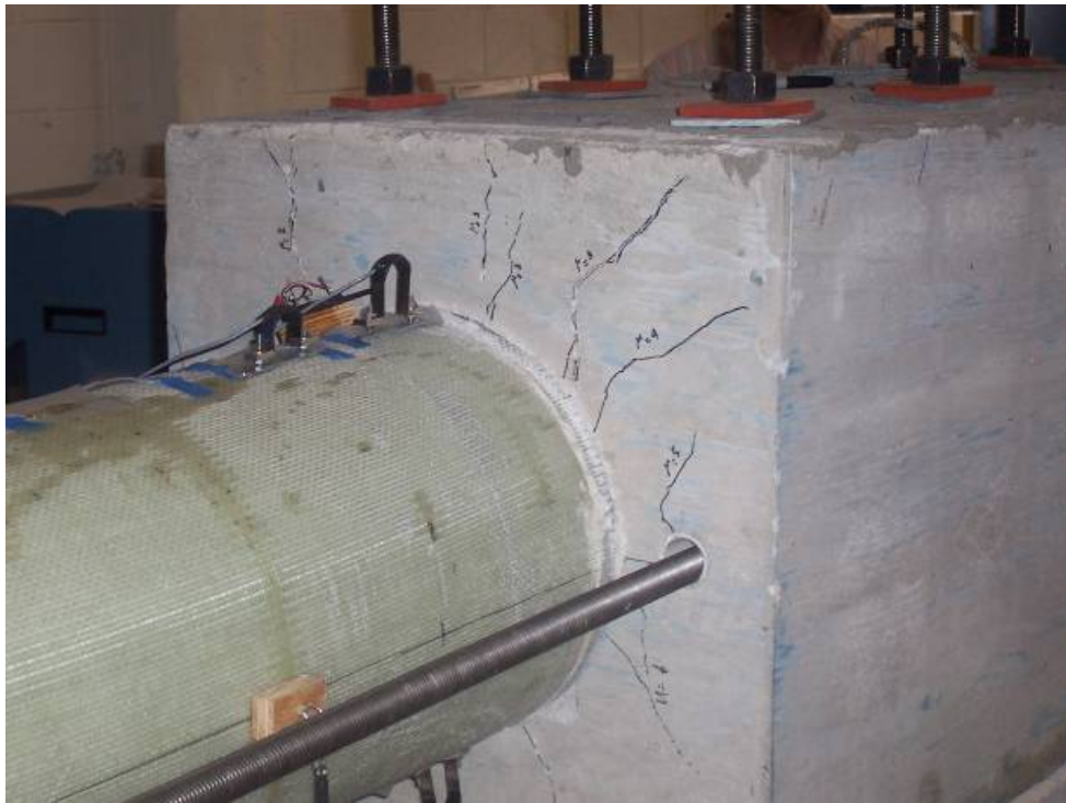
Figure 3.35 Footing Cracks in Specimen G
