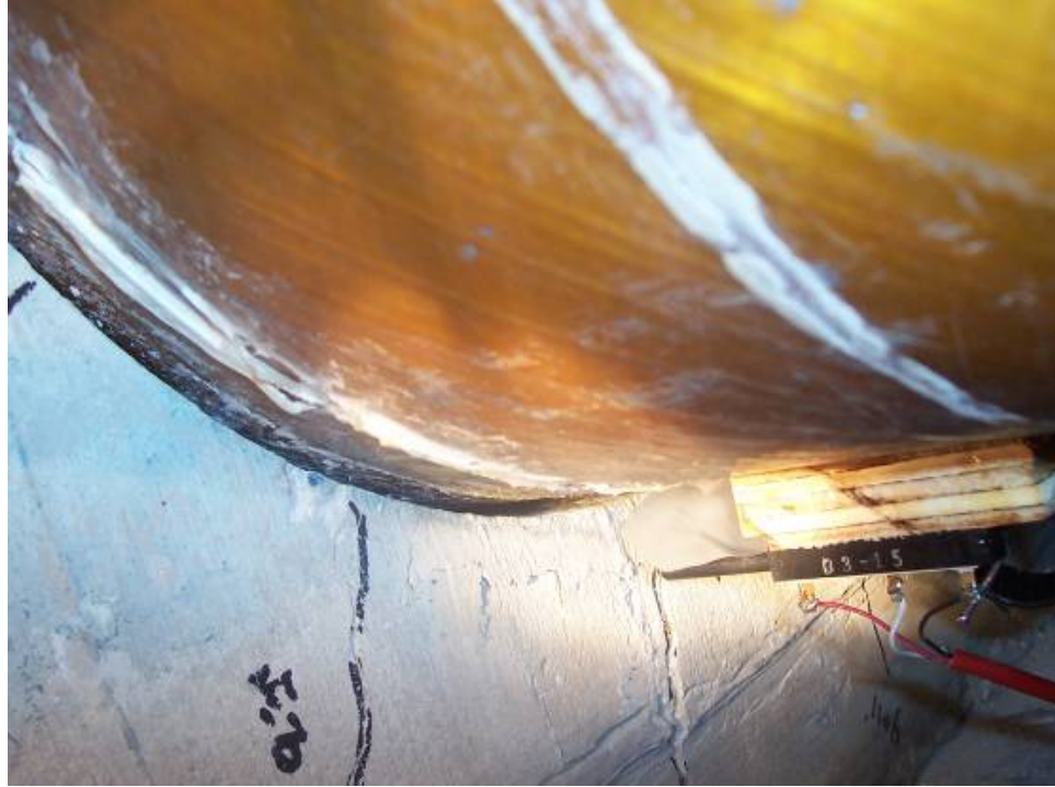
Figure 3.38 Separation between FRP Tube and RC Footing in Specimen Y
