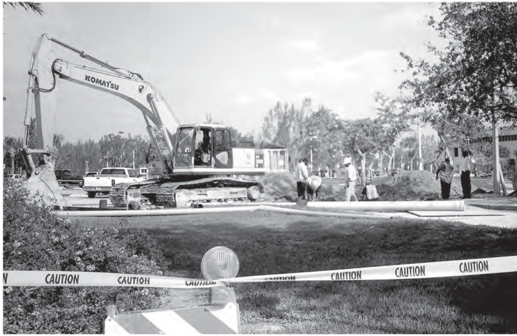
WORK SITE: Construction crews continue to work on a sewage and water hook-up for the new Marine Biology building and the Wolfe University Center. Vice Provost Raul Moncarz estimates the work will be completed within the next four weeks. BETSY MARTINEZ/THE BEACON
