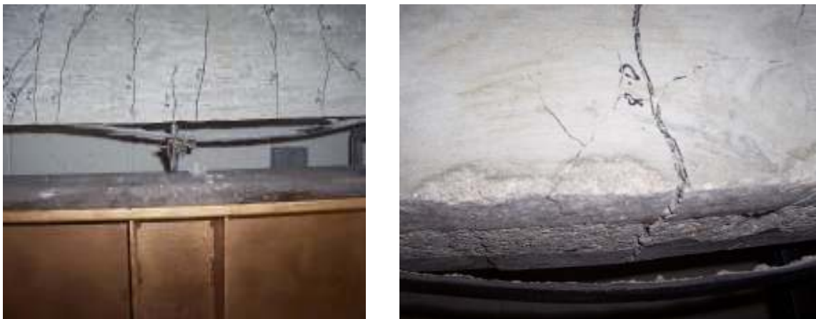
Figure 3.24 Typical Failure Mode for the Pre-Cured FRP Specimens with Different Surface Roughness
