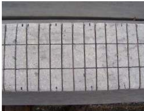
Figure 3.14 Typical Crack Profile with 1 in. Spacing
