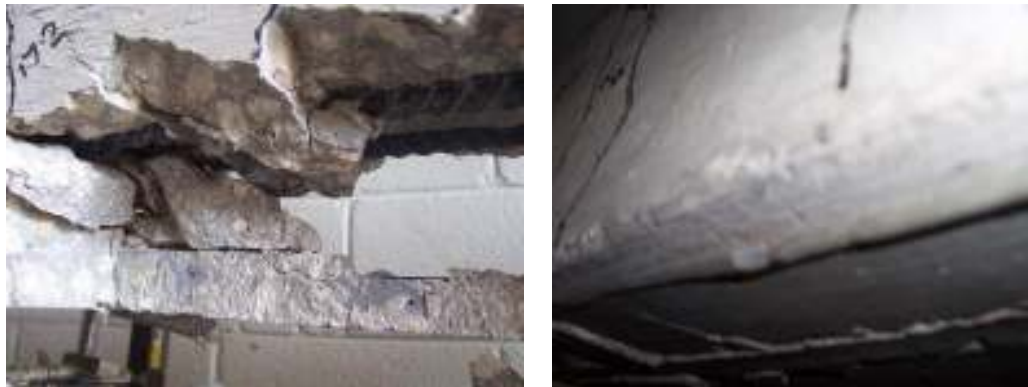
(a) Concrete Splitting (b) Epoxy Splitting Figure 3.65 Failure Mode of Undersized Groove Specimens (NSM Strip)
