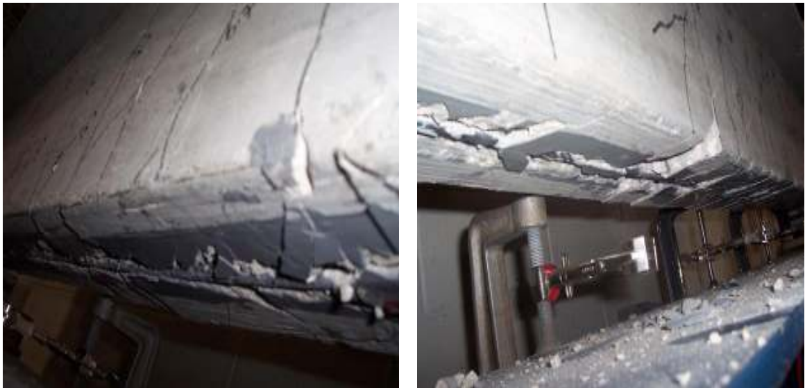
Figure 3.76 Failure Mode of Undersized Specimens (NSM Bar)
