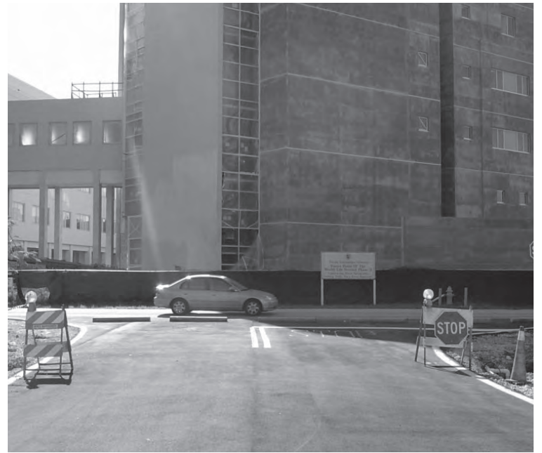
WHAT GIVES?: The new entrance to the University Park Apartments is still under construction for no obvious reason. JONATHAN BANKE / THE BEACON
