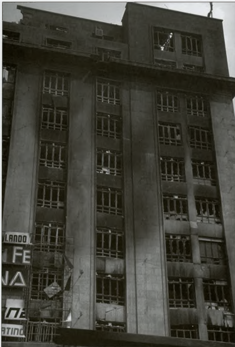
Mexico City's famous Hotel Regis, in shambles after the massive earthquake of September 19, 1985, which measured 8.10. Photo: Steinbrugge Collection, EERC.
