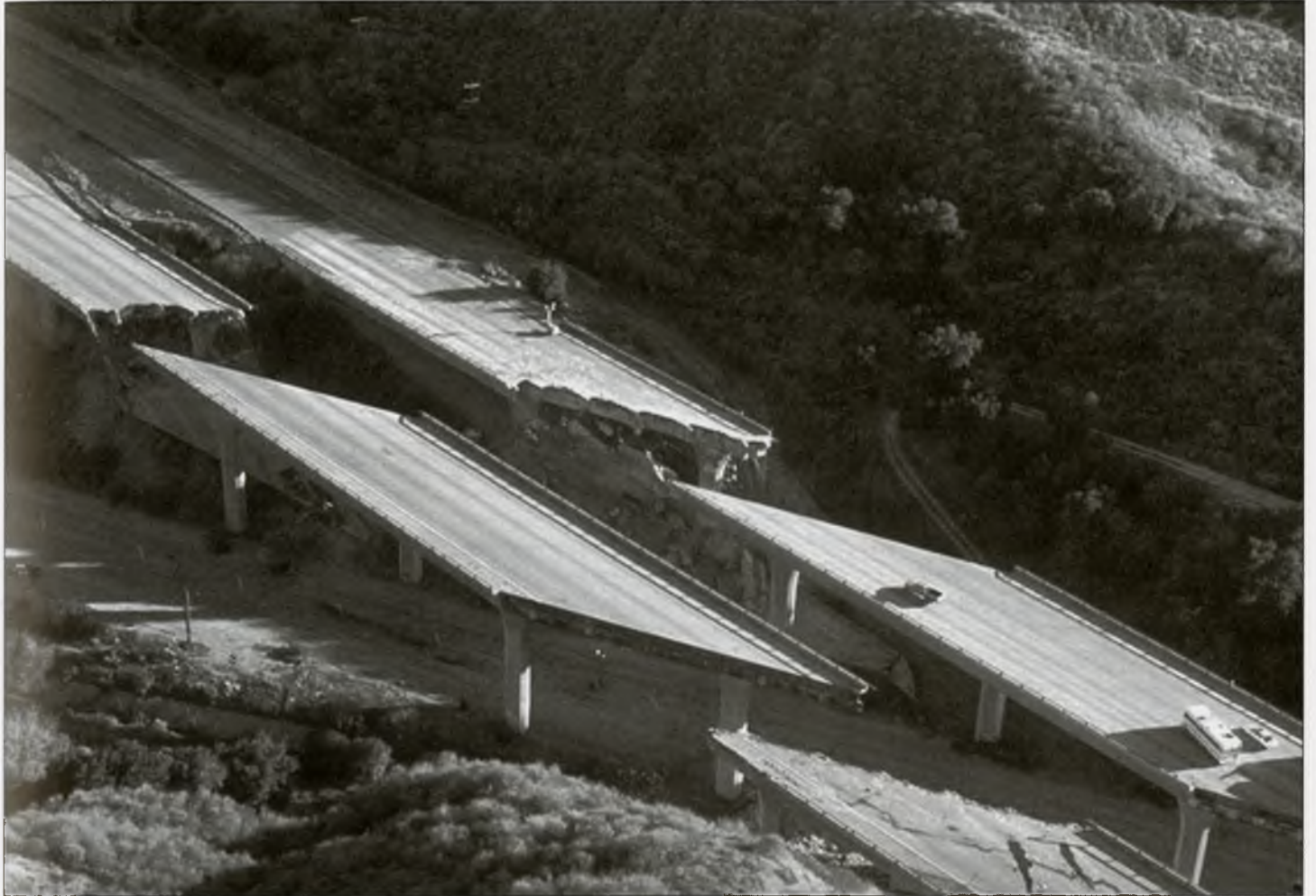
Aerial view of the collapse of Interstate 5 at Gavin Canyon, California. Extensive damage was inflicted on infrastructure as a result of the January 17, 1994, earthquake in Northridge, California, which measured 6.69. This natural disaster has proven to be the costliest in US history—surpassing Hurricane Andrew. Photo: Northridge Collection, EERC.
