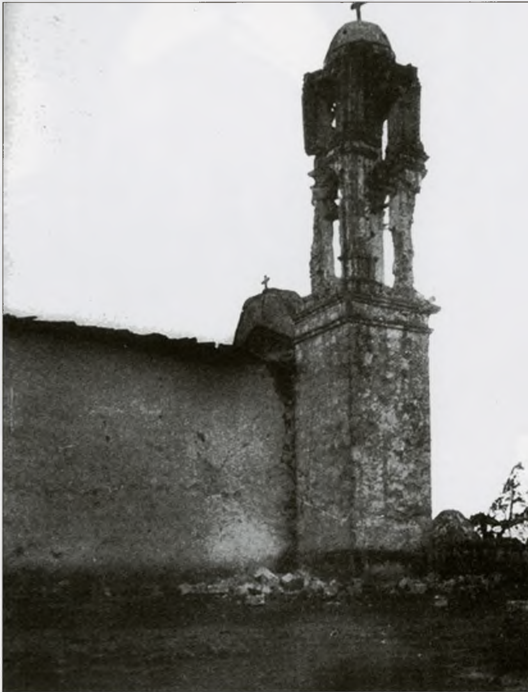
The crumbling tower of the Church of San Juan de los Jarros, damaged by the earthquake that shook Acambay, Mexico, on November 19, 1912. The quake registered a magnitude of 7.80. Photo: Steinbrugge Collection, EERC.
