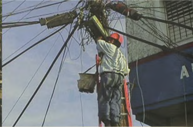
Pirating electricity is a common practice in the developing world, and the pirates make a good living. Unfortunately for the power company workers, like this one in Santo Domingo, they have to sort through the highly charged mess.
