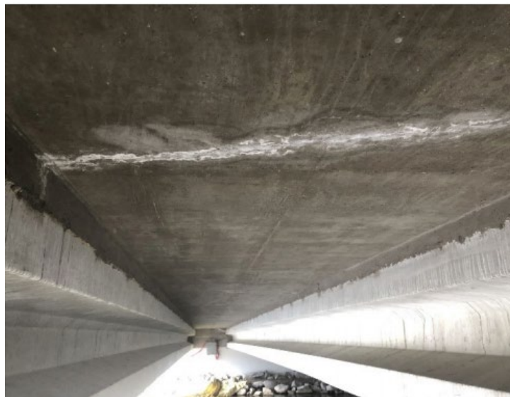
Figure 29 Full depth crack in GFRP reinforced bridge deck (Shafei 2023)
