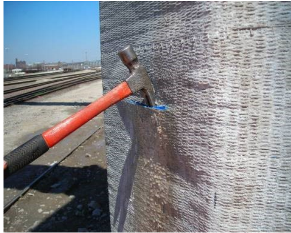
Figure 39 Rupture due to moisture entrapment (Source: Authors)
