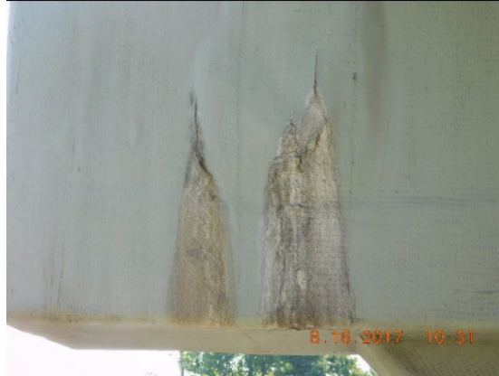
Figure 41 FRP discoloration (Pevey et al. 2021)
