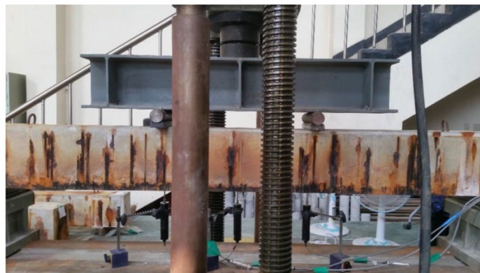
Figure 48 Rust stains indicating corrosion of steel reinforcement in concrete substrate (Jung, Jeong, and Lee 2022)
