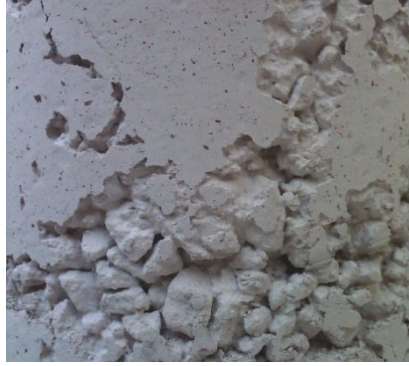
Figure 23 Concrete voids (Source: Authors)
