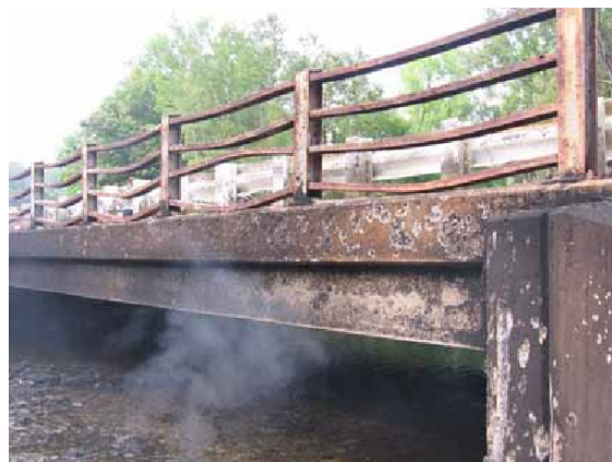
Figure 52 Fire damage (Graybeal 2007)
