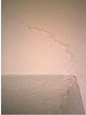
Figure 38 Cracks (Source: Authors)
