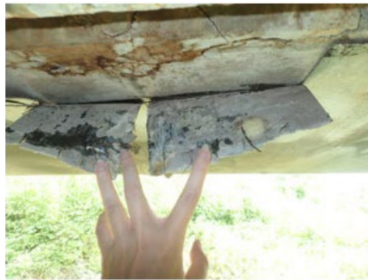
Figure 43 End peeling (Baniya et al. 2022)
