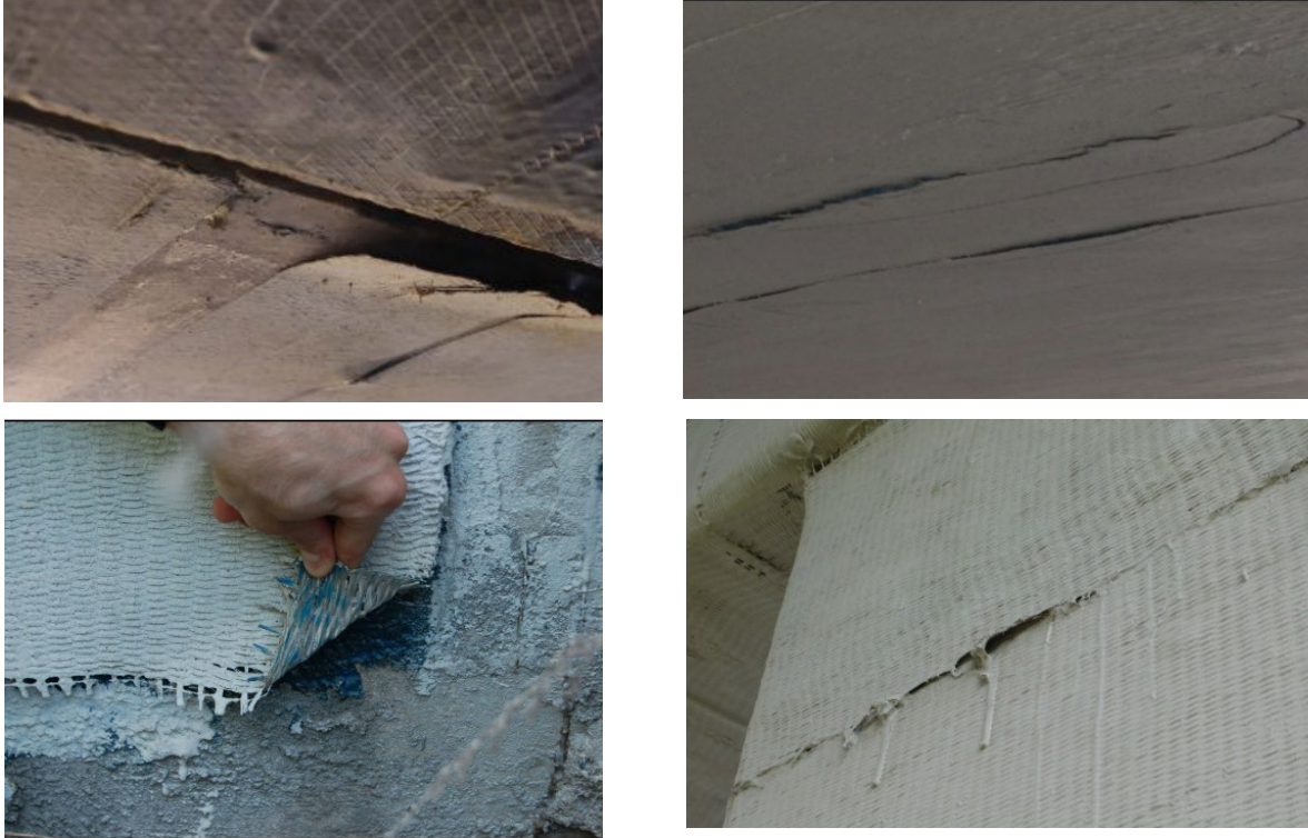
Figure 42 Debonding (Baniya et al. 2022; Pevey et al. 2021)
