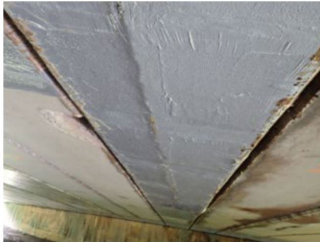
Figure 47 Bulged CFRP layer indicating the presence of a longitudinal crack beneath (Baniya et al. 2022)
