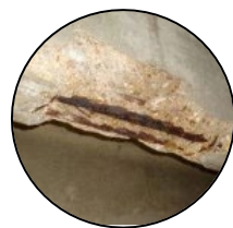
F.2 Steel Corrosion
